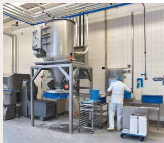
Example of an application in the Food & Beverage Industry: the user needed a full stainless steel 22mm drop in a wash down zone.
